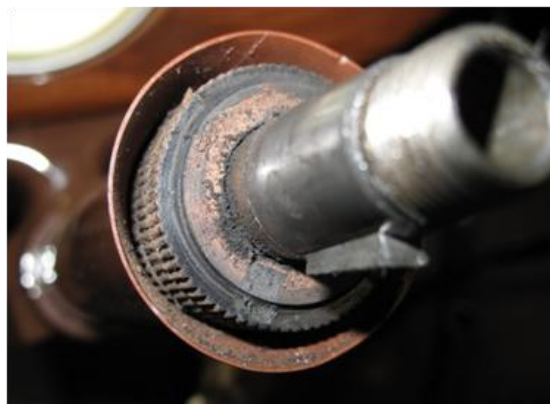
Old bushing still in place – looks like it should have been pushed in further – note how the material has deteriorated
